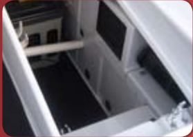
Heaters above water tanks
